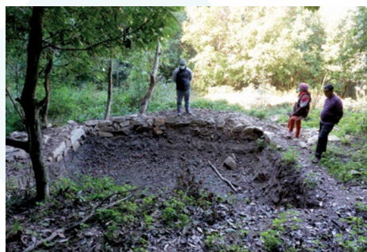
Recharge pits and ponds for natural groundwater percolation to overcome water scarcity.
